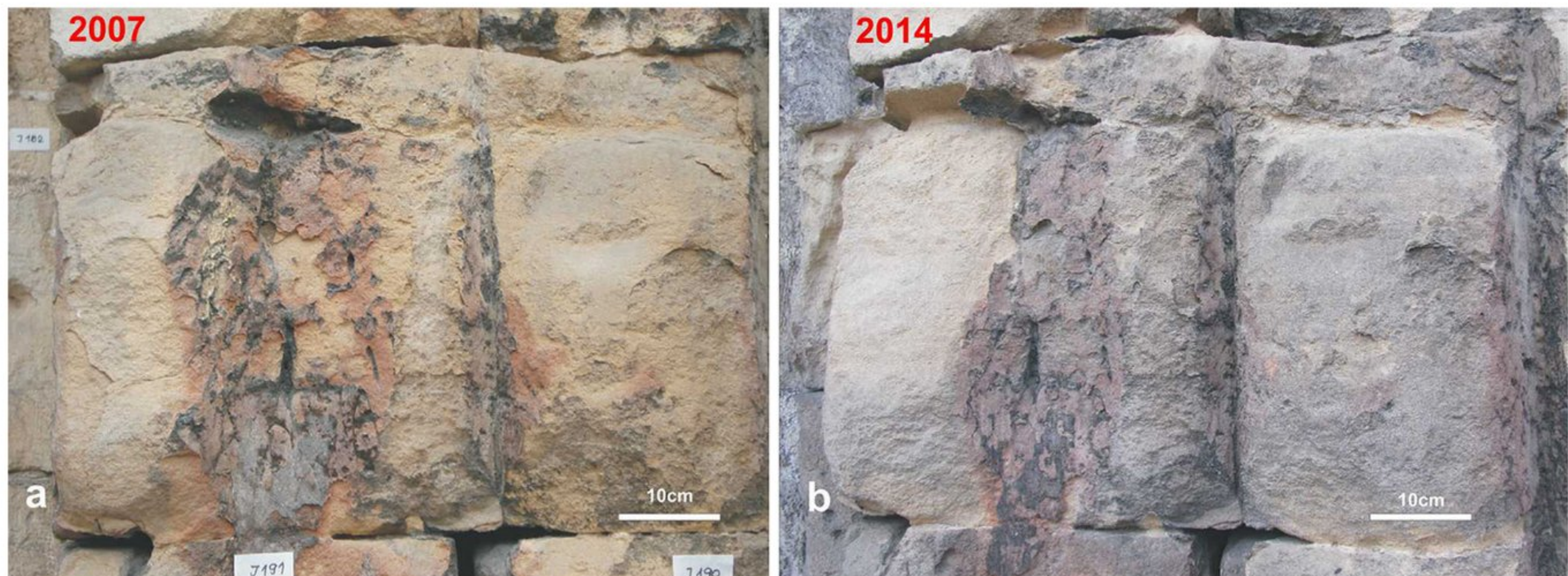
Fig. 9 Evident increase of stone decay on southern façade of the Dark Gate
