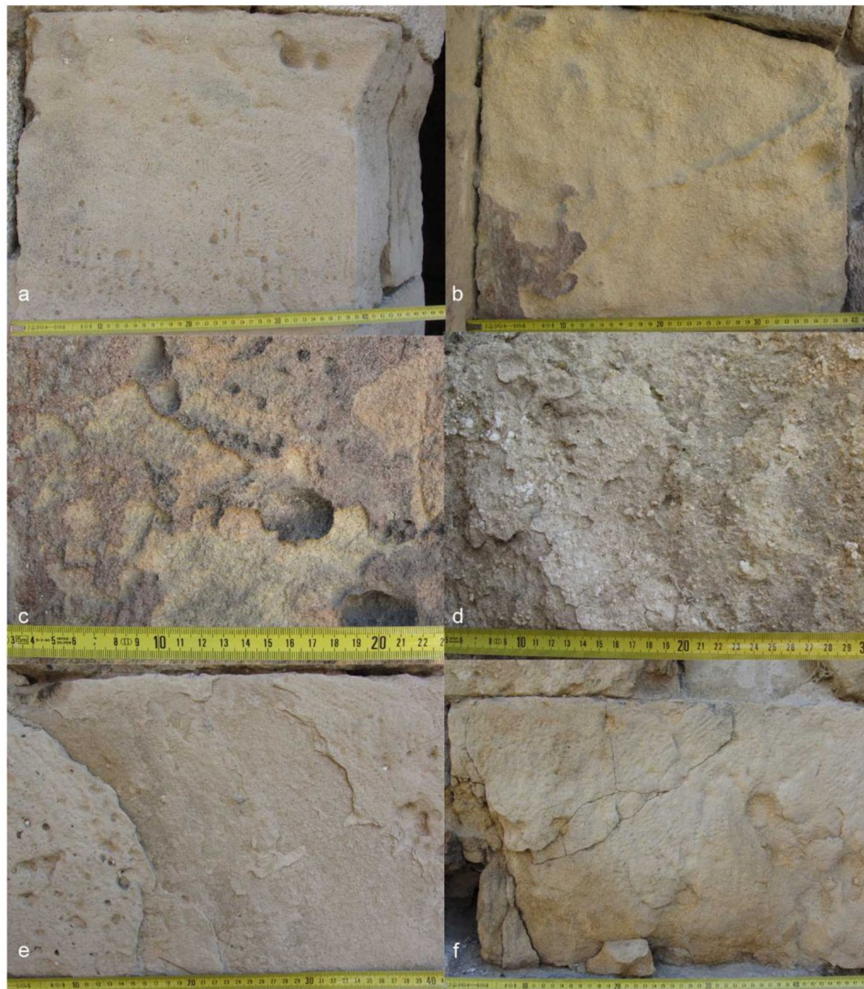
Fig. 4 Weathering forms on the Dark Gate: a relief, b surface recession and granular disintegration, c remains of black crust, discoloration and detachment of crusts with stone material, d Surface
