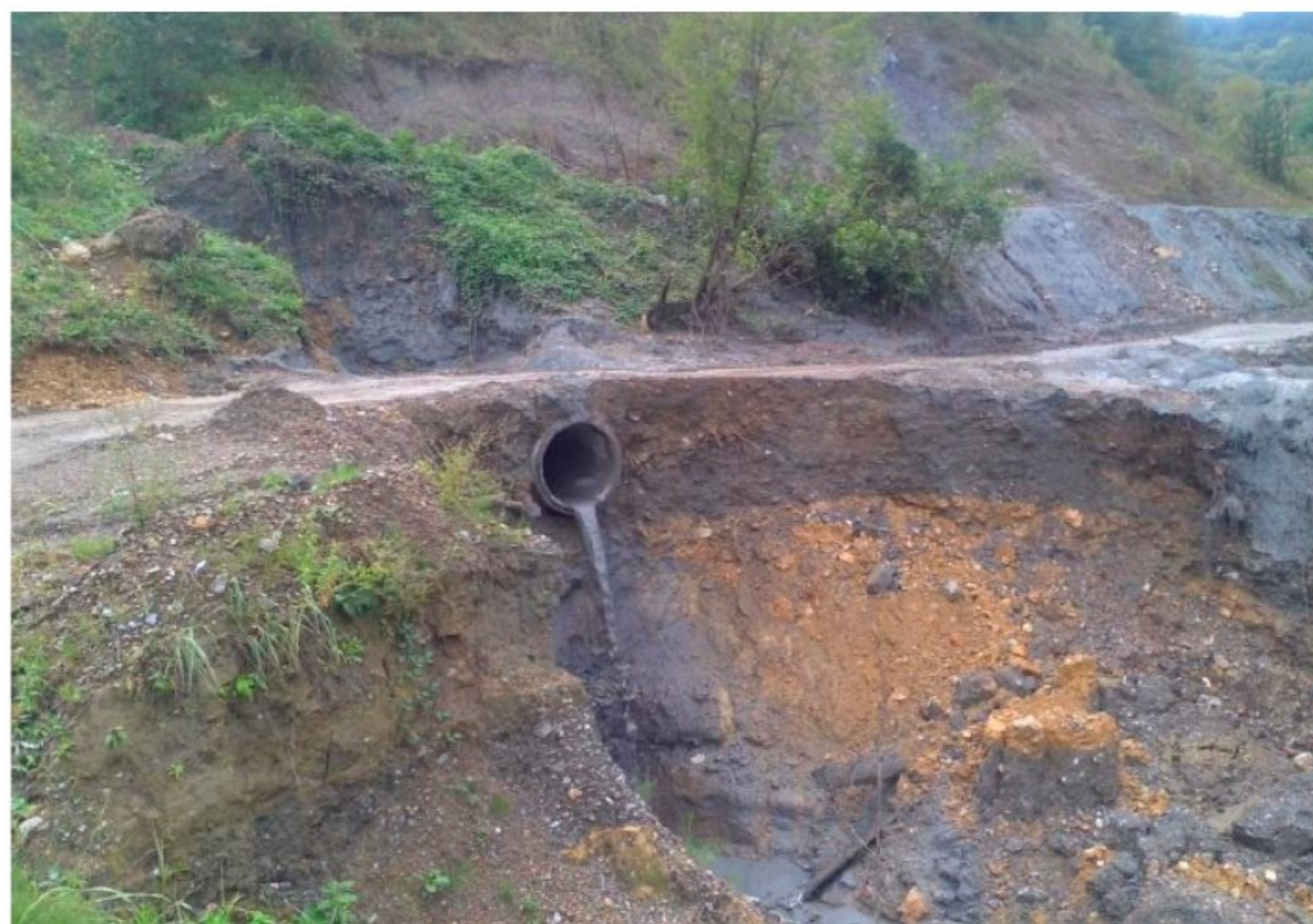
Figure 5. The damaged pipe culvert on the western field. Reproduced with permission from the Water Institute “Jaroslav Černí” [10].
