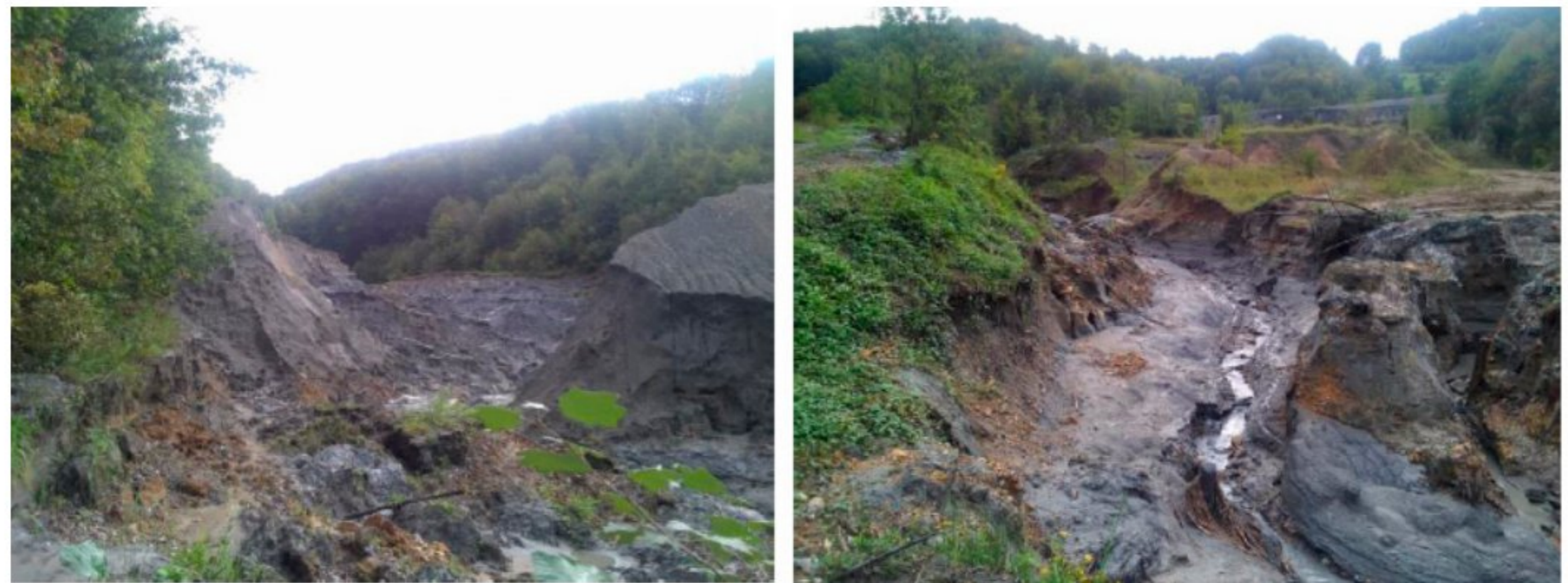
Figure 4. The damaged embankment of the eastern field. Reproduced with permission from the Water Institute “Jaroslav Černí” [10].
