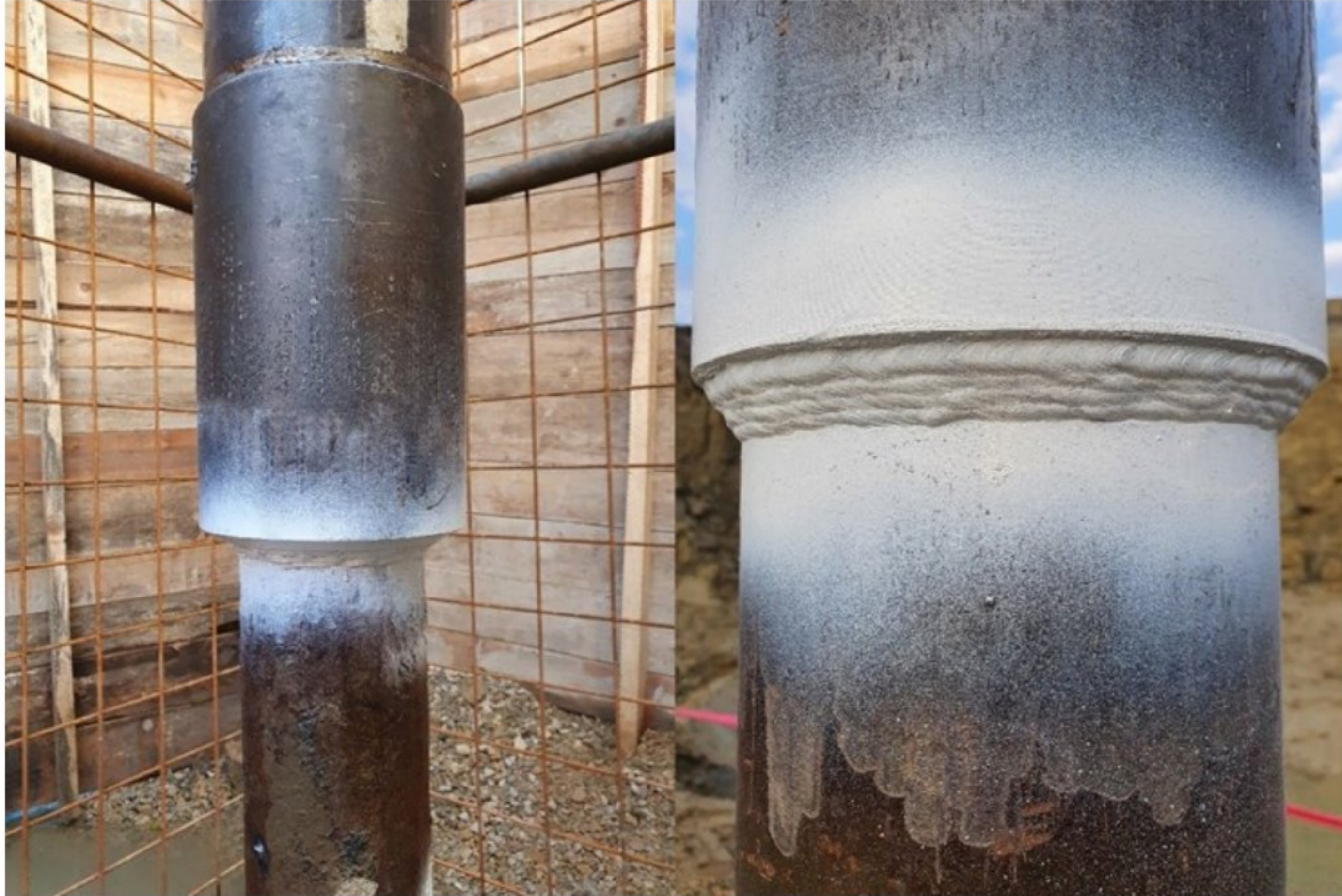
Figure 4 A detailed view of the welded production casing
